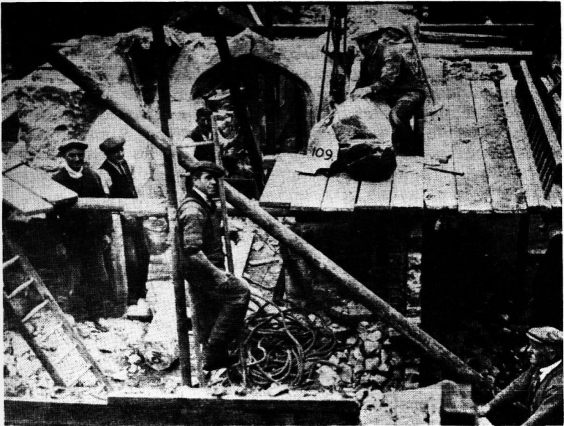
Fig. 2 The porch in course of dismantling (Photo: Macclesfield Sunday School Heritage Centre)
